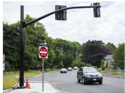
Black Intersection Mast Arms
