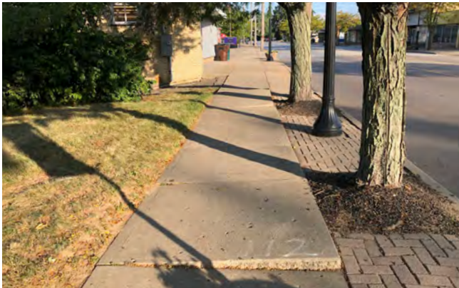
Current sidewalk conditions in the Mt. Airy NBD in the 5500 Block of Colerain Avenue
